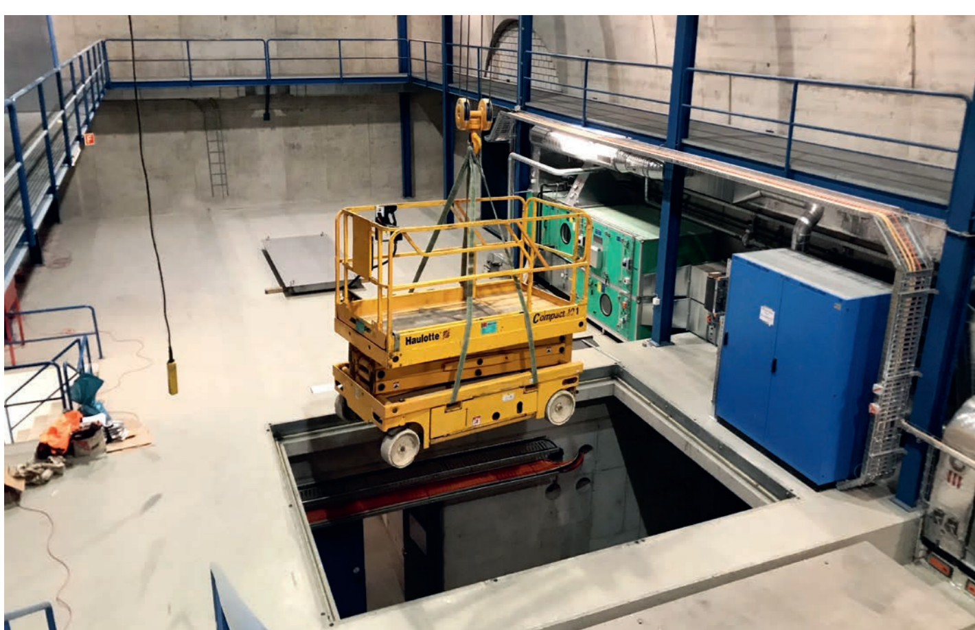
Installation in Zentrale
